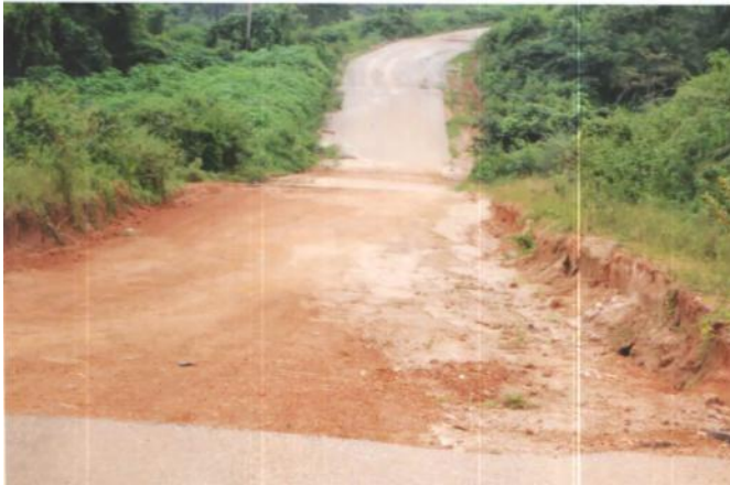
Plate 9: Failed Segment of road along Eyio and Awo Source: Field survey, 2020
