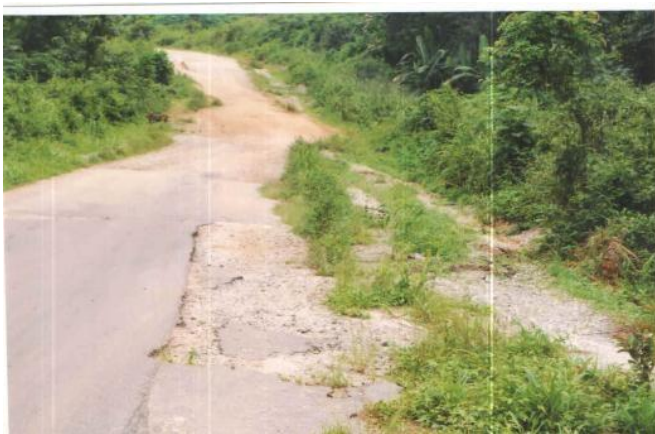
Plate 6: Failed Segment of Road between Esure and Eyio
