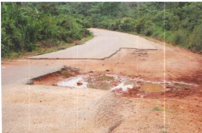
Plate 7: Failed Segment of road along Esure-Eyio-Awo road
