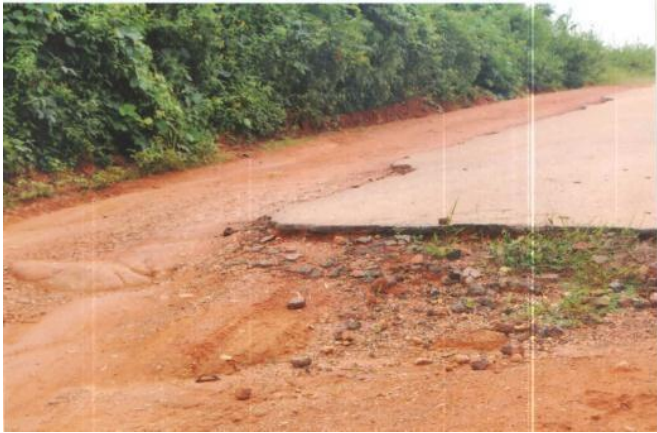
Plate 8: Failed Segment of road along Are-Afao-Igbemo road Source: Field survey, 2020
