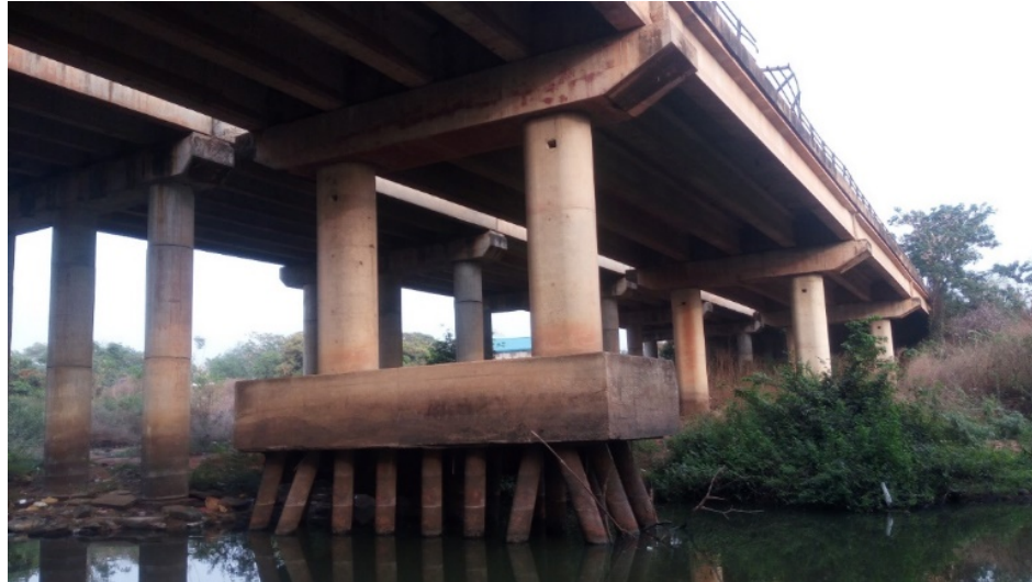
Fig. 1 Asa-Dam Bridge showing signs of scouring
